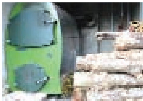
Wood log central heating boiler
