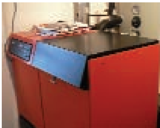
Wood pellet central heating boiler
