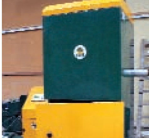
Wood chip central heating boiler
