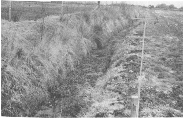
Figure 10. Aging of a drainage system is inevitable as nature tends to level both humps and hollows. The drain shown above is at a gentle gradient. The accumulation of weeds will reduce water velocity allowing deposition of silt. The drain will need to be cleaned using a hydraulic machine every 5–10 years.
