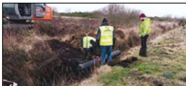
Plastic dam being installed on Case Study Farm A on 7th Feb 2023
