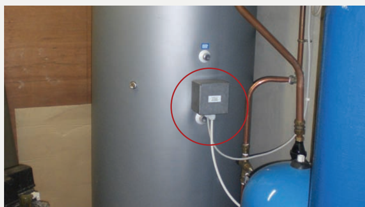
FIGURE 1: Typical location of an immersion element in a 500L water tank.
