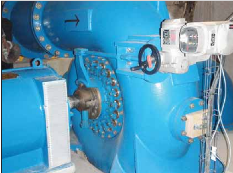
Turbine installed in Donegal – Source D Twomey
