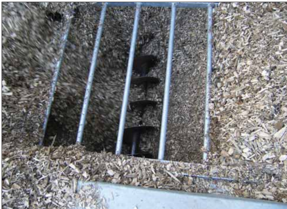
Wood chip being fed through and auger system to the boiler.
