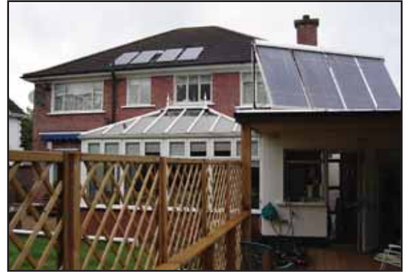
Solar PV panels – Source Efgem
