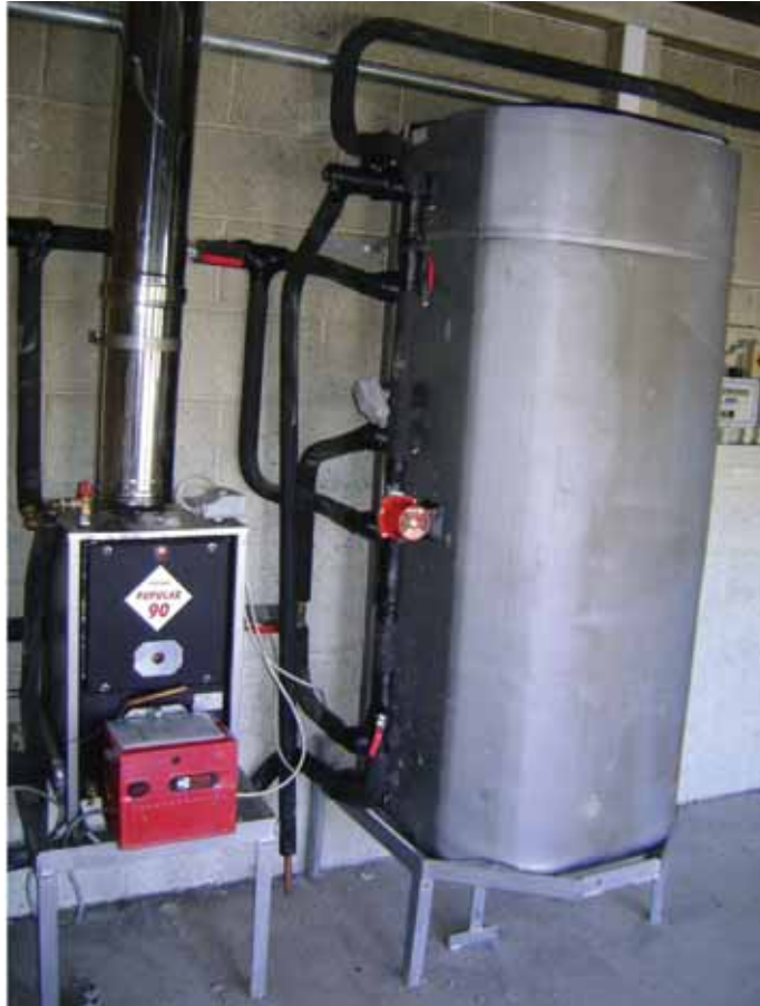
26.4 kW oil fired burner running on kerosene
