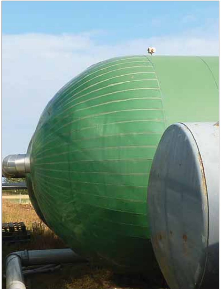
Well insulated heat storage tanks are essential to reduce the cost of CO 2 enrichment
