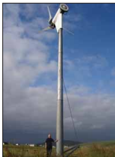
Small scale 6 kW wind turbine - Source Efgem.
