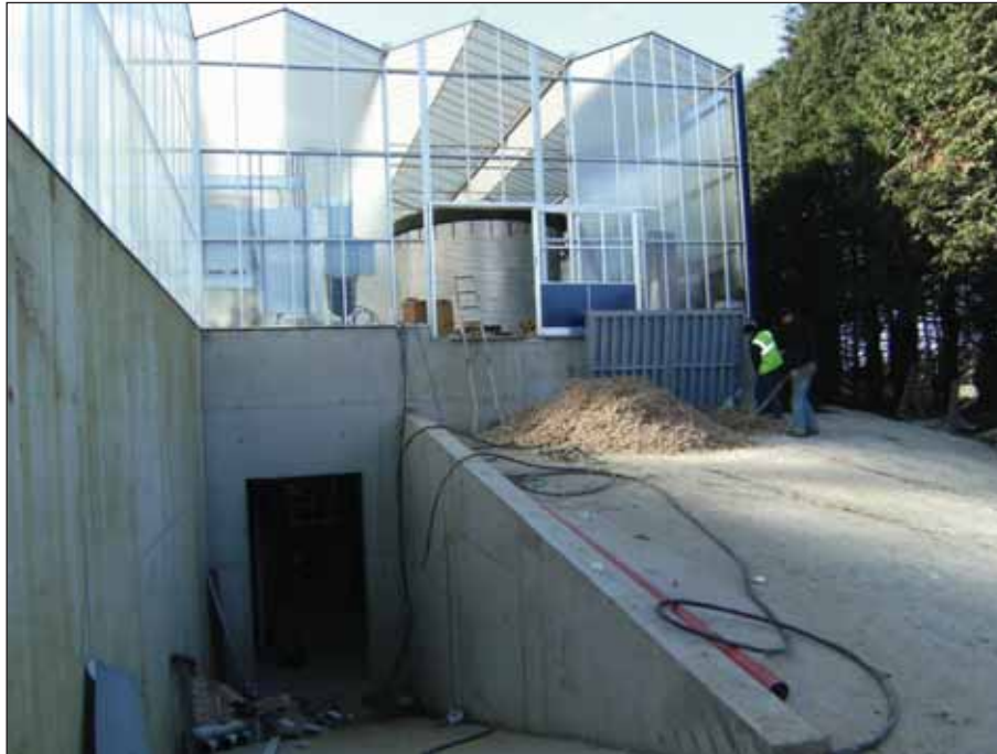
A wood chip boiler heating a 0.8 ha glasshouse which grow bedding and pot plants outside Gorey in Co. Wexford. The wood chip is stored above and gravity fed by auger into the boiler in the bunker below.
