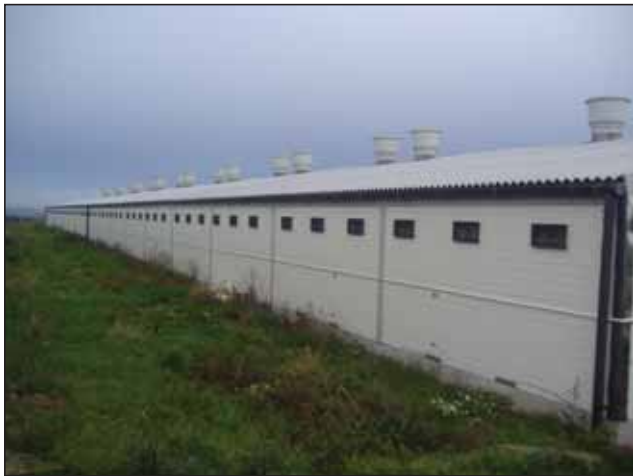
External view of Natural Power ventilated finishing house. Air inlets to the side and warm exits through roof mounted outlets.
