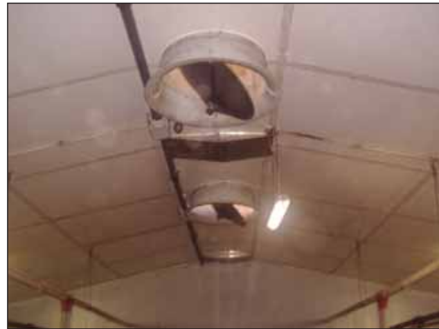
Internal view of outlets for Natural Power ventilated house.
