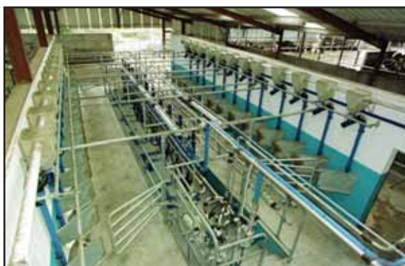
Annual savings can be made on dairy farms by monitoring energy consumption and putting in place a number of good house keeping measures.
