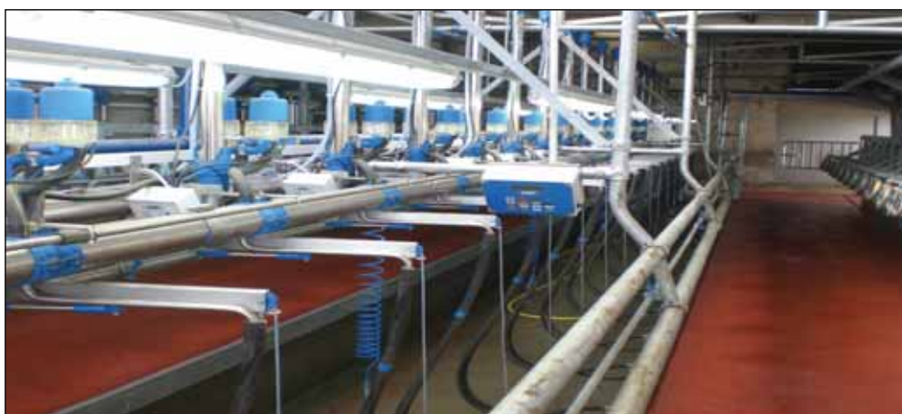
Well lit parlour with 2 rows of double fluorescent fittings
