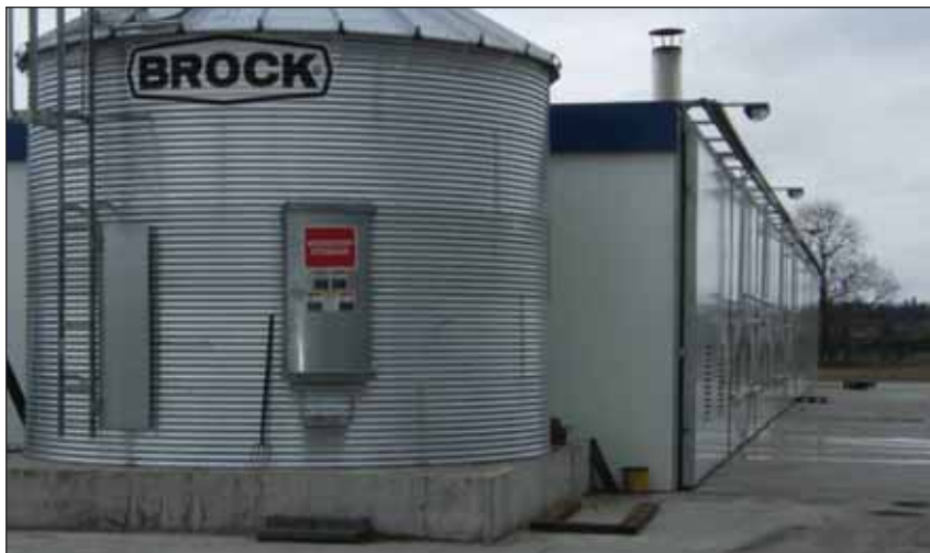
1 MW Wood pellet boiler and storage facility on a mushroom farm outside Tullow, Carlow. The boiler produces heat for the mushroom house at 18°C and 25°C depending on cycle and it also provides steam to 'Steam Out' houses after growing cycle.
