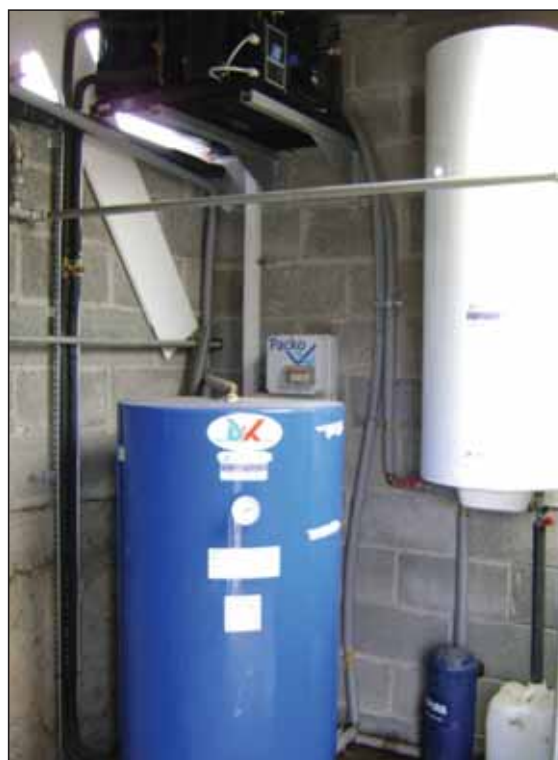
Heat Recovery System
