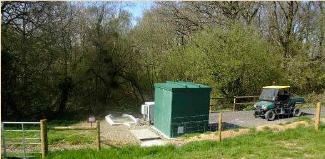
Flume area – accessed by service tracks
