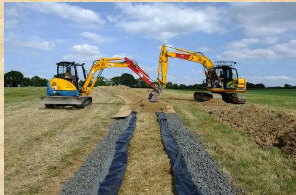
Back-to-back French Drains on watersheds
