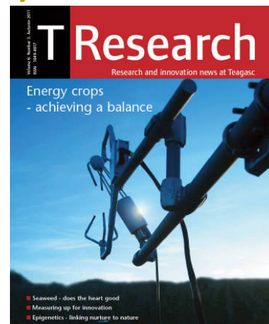
The field-scale CO 2 eddy covariance monitoring equipment at Johnstown Castle, Wexford
