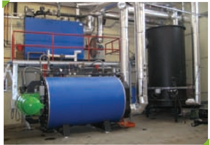
Figure 2: Biomass CHP plant at Oak Park featuring the gasifier (black cylinder on right), gas combustion chamber (blue cylinder in the centre) and the Stirling engine (green unit attached to the combustion chamber).
