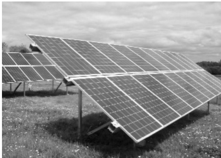
Figure 1 Free standing PV array in Co Fermanagh
