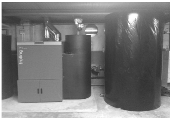
Figure 1 Froling 99 kWh pellet boiler
