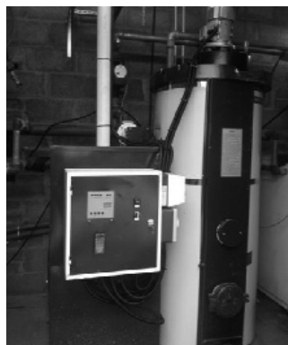
Figure 2 99 kWh Chinese pellet boiler
