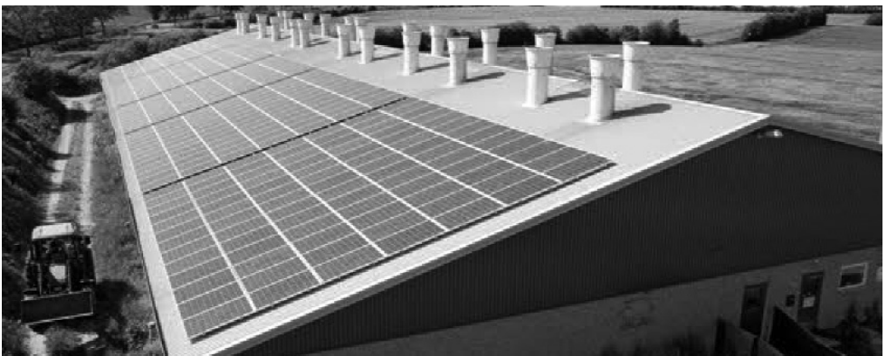
Figure 2 PV on pig house roof
