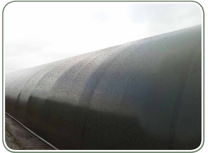
14. Compost dust on a growing tunnel roof after emptying reinforces the importance of effective end of crop steam cook-out
