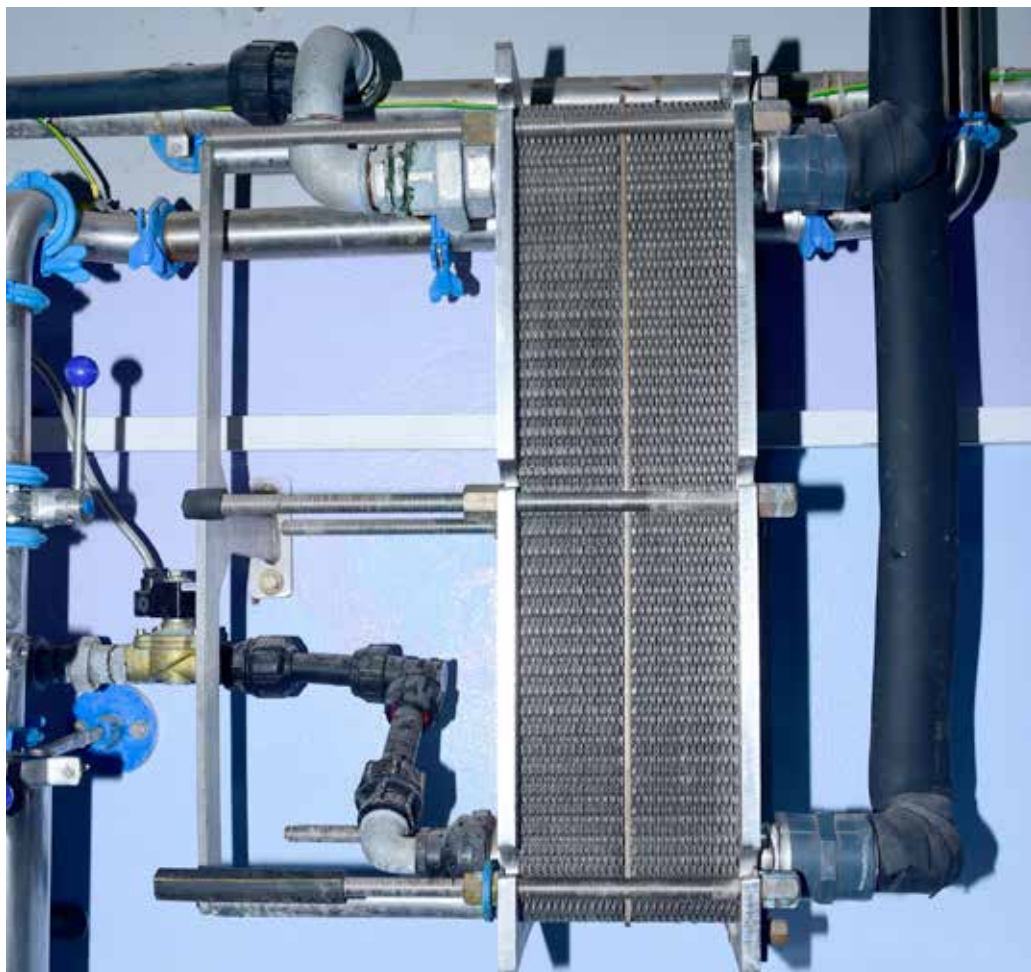
Picture 21. Dual stage plate cooler fitted with solenoid valve on the water pipe
