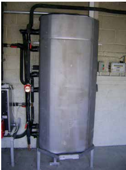
Picture 22. Insulated hot water tank with insulation on all water transfer pipework
