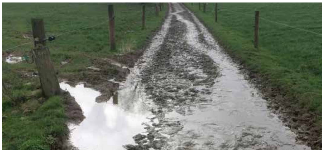
Picture 4. Water trapped on the roadway lodges at low points. The photograph shows the most vulnerable first 100 m of this farm roadway. The cows are following tracks due to a less than perfect surface
